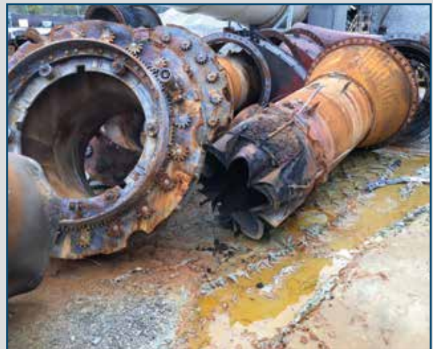
UNCHECKED PROBLEMS LEAD TO SYSTEM FAILURE
